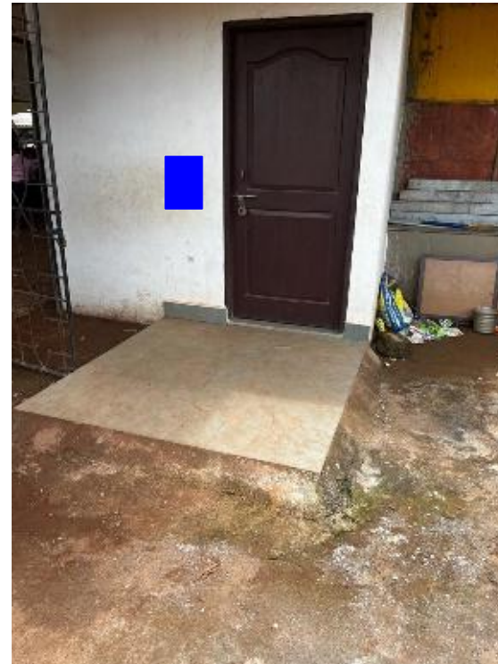
Accessible room signage not provided.
