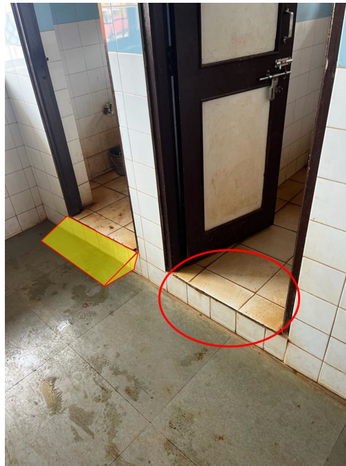
There are level differences at door openings.
