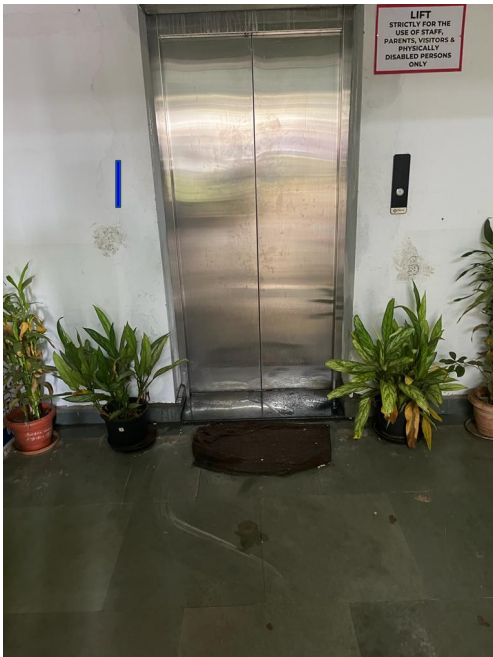
Signage in the lift not as per standards.
