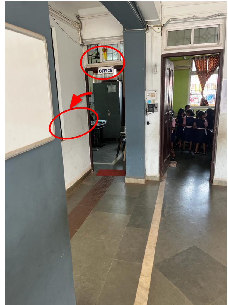
SIGNAGE ALL AROUND THE CAMPUS IS NOT PROVIDED IN BRAILLE. THERE IS INSUFFICIENT DIRECTIONAL SIGNAGE
