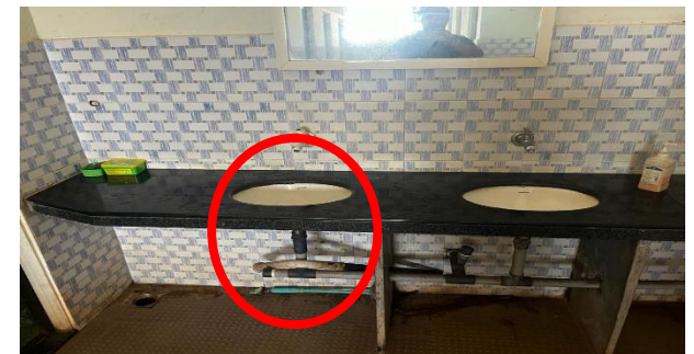
Basins and urinals not provided at HG standard height
