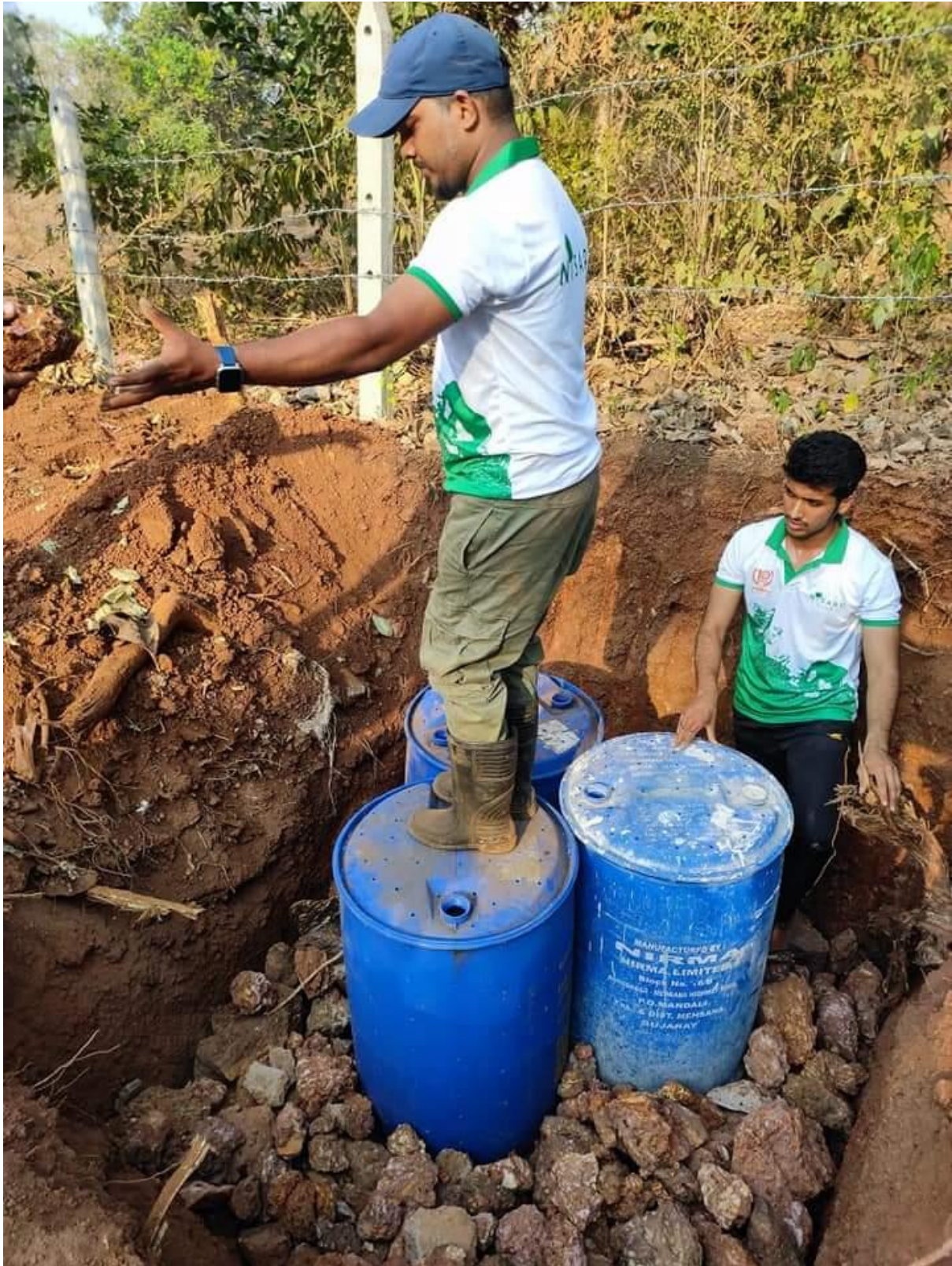
Rainwater Recharge Unit being set up by faculty and students of the college
