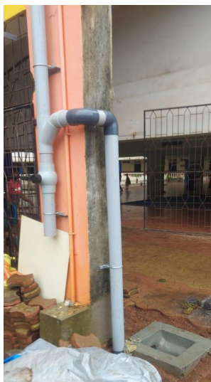
Fig 5: First rain separator
